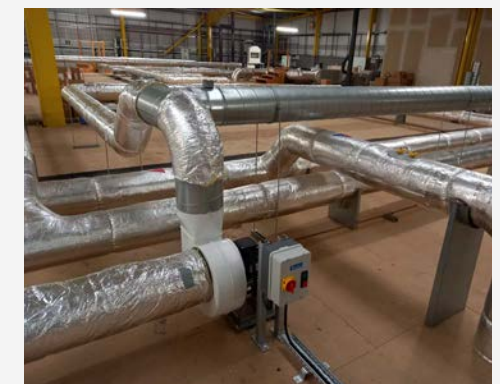
Wakefield, UK, Redirected ducting
